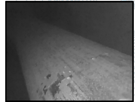
With HydroFLOW Thin layer of loose scale
