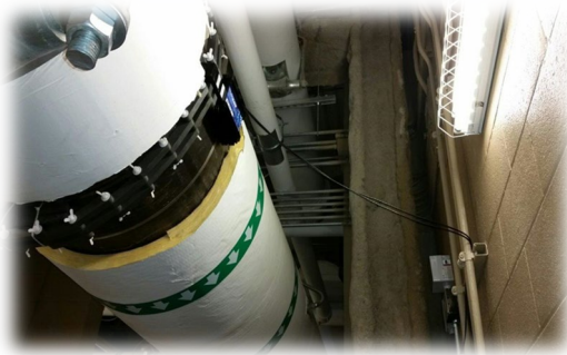
30" line between chiller and cooling tower, Hollywood Casino, Columbus, OH
