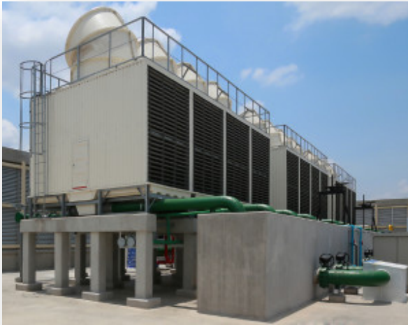
Cooling Towers / Boilers / Pools
